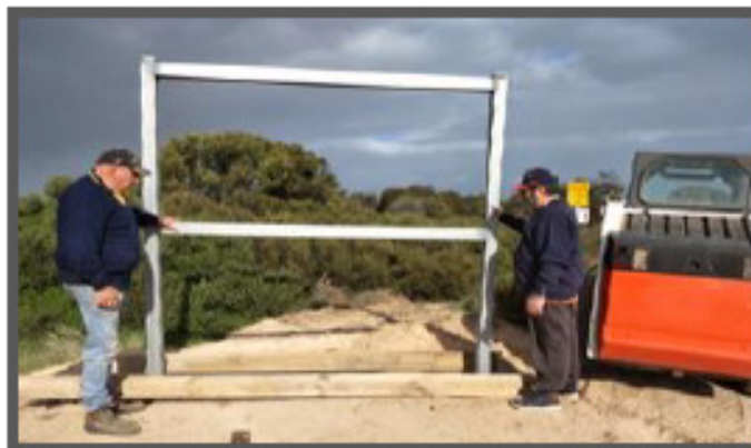
Herman Wyten and Ian Marschall cementing in frame work for new "Welcome to Balgowan" sign.
